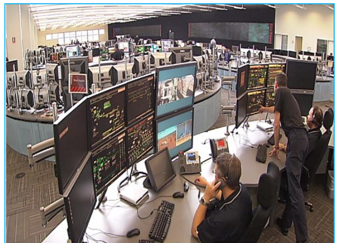
Control room, located in Perth, for remote mining operations 1500 kilometres away. Image courtesy of Rio Tinto.
