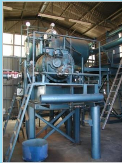
Geothermal equipment at Birdsville. Image courtesy of Ergon Energy
